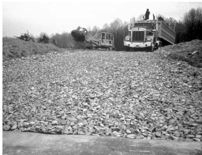
Stabilized construction entrances allow dirt to be removed from tire treads as trucks leave construction sites.
